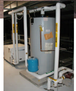
WATER TO WATER HEAT PUMP FOR DOMESTIC WATER
