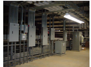
ELECTRICAL IN MEZZANINE
